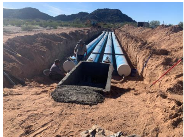
FIGURE 4. This type of system, which consists of a series of large PVC tubes or pipes that feed the drinker virtually eliminates maintenance and improves water availability for desert bighorn sheep.
