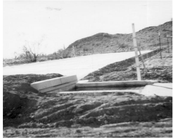
FIGURE 3. An apron and vault-type bighorn sheep development offered improvements from the tinaja water source as evaporation was minimized. A disadvantage of this type of catchment was that the apron required considerable maintenance to ensure functionality.
